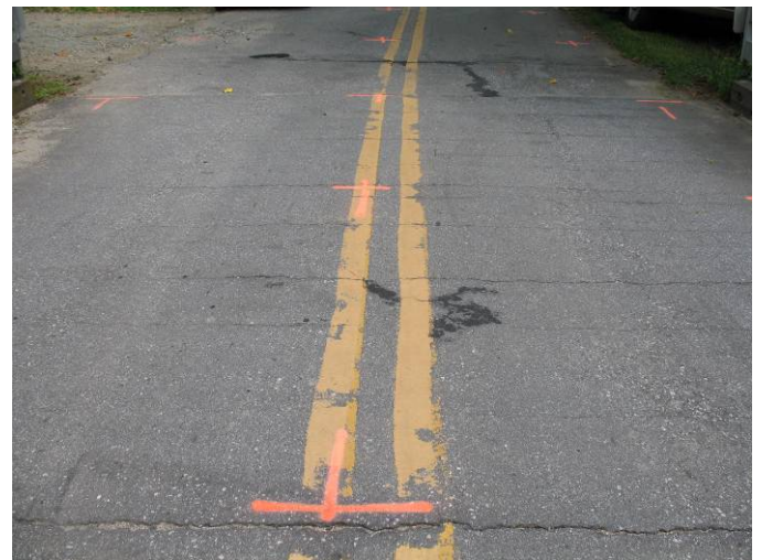
Figure 107. Presence of Transverse Cracks
