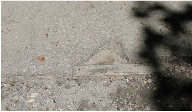
Figure 13. Pavement Chipping at West End
