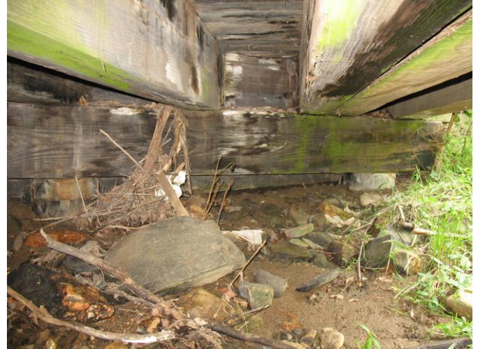
Figure 198. Fungal Growth throughout Superstructure
