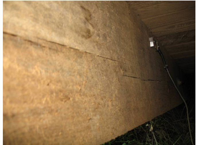
Figure 74. Observed Checking in Girders
