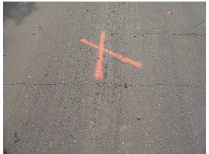
Figure 42. Pavement Chipping at West End
