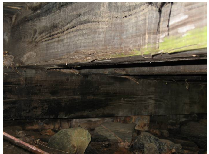
Figure 199. Mechanical Damage to Girder
