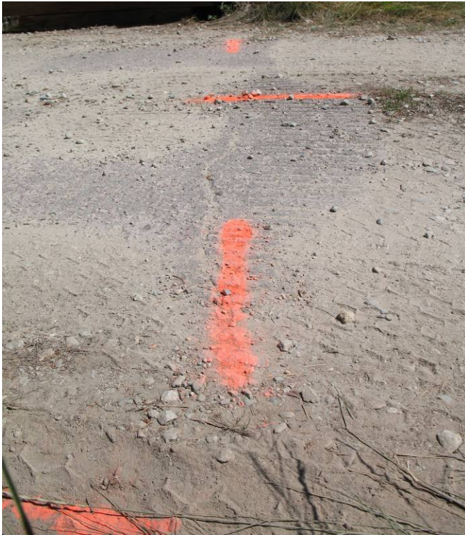
Figure 439. Wearing Surface Cracking and Debris
