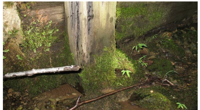
Figure 15. Moss Growth at Base of Substructure Posts
