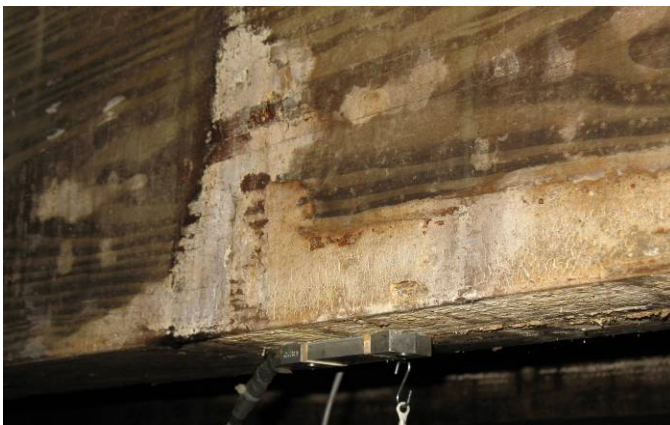
Figure 14. Biotic Growth on Girders
