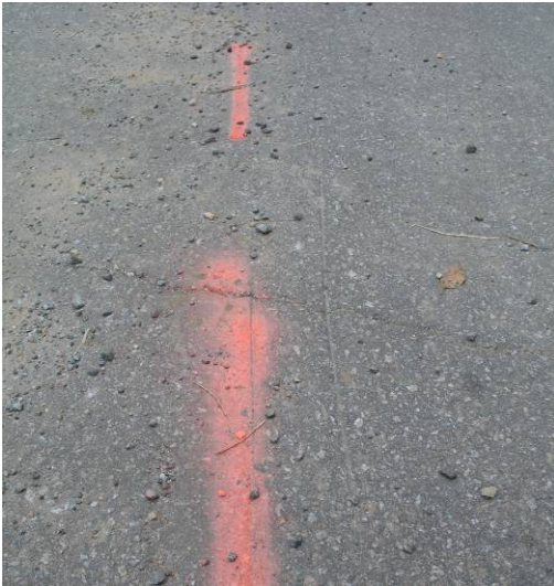
Figure 167. Minor Transverse Cracks
