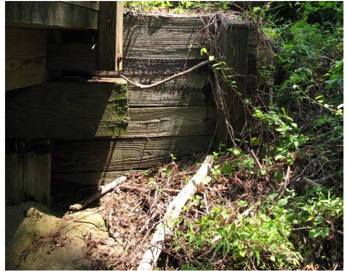
Figure 230. Wingwall Weathering and Decay
