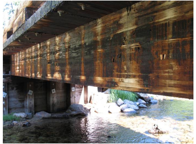
Figure 441. Girder Streaking and Holes
