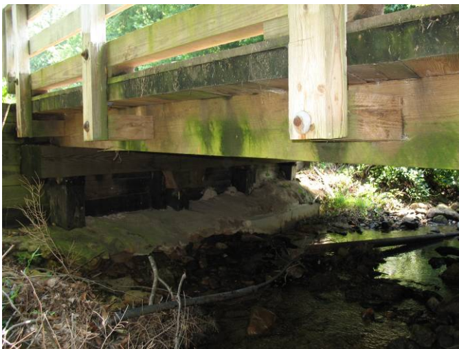
Figure 229. Moss Growth on Girder 19
