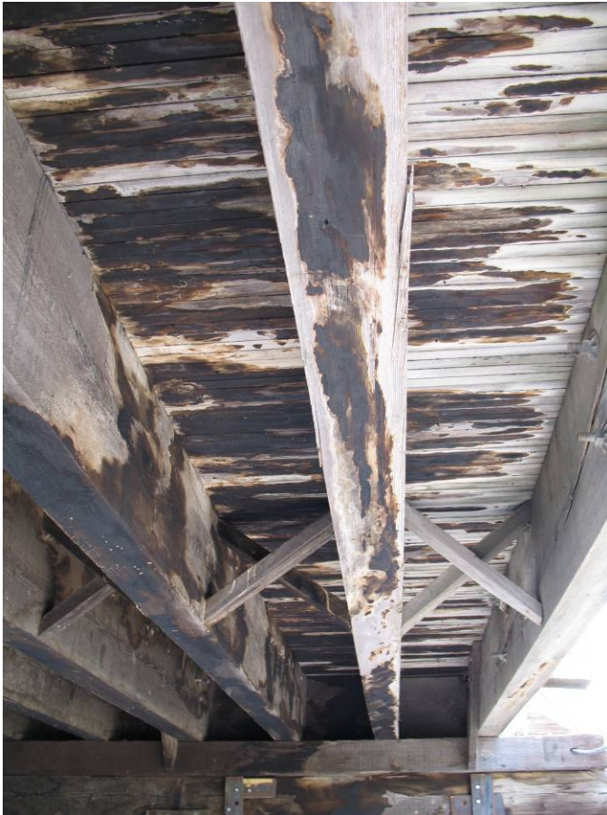
Figure 377. White Residue Formation on Deck
