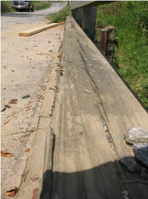
Figure 169. Advanced Degradation throughout Curbs
