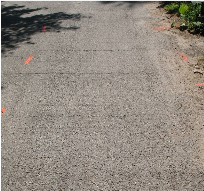
Figure 137. Transverse Cracks in the Wearing Surface Deck
