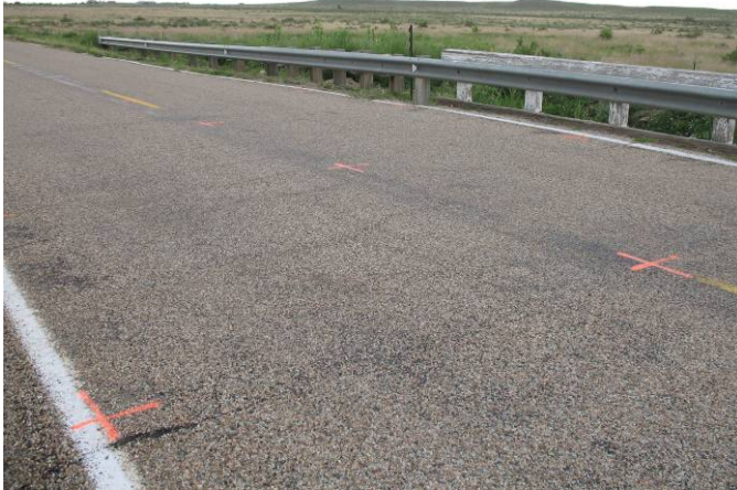
Figure 314. Transverse Wearing Surface Cracking
