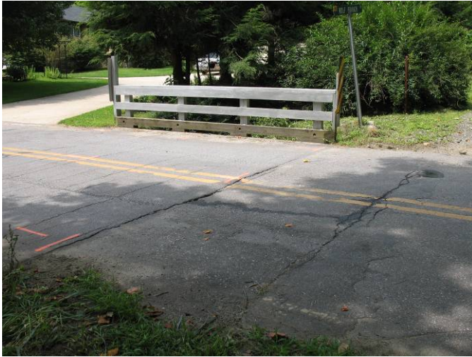
Figure 108. Transverse Cracks at Bridge Approach
