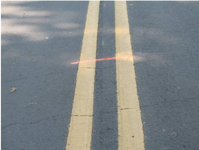
Figure 228. Observed Transverse Cracks
