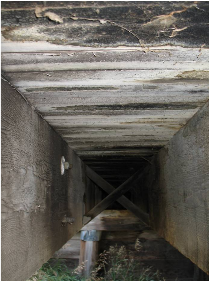
Figure 349. White Residue Formation on Deck
