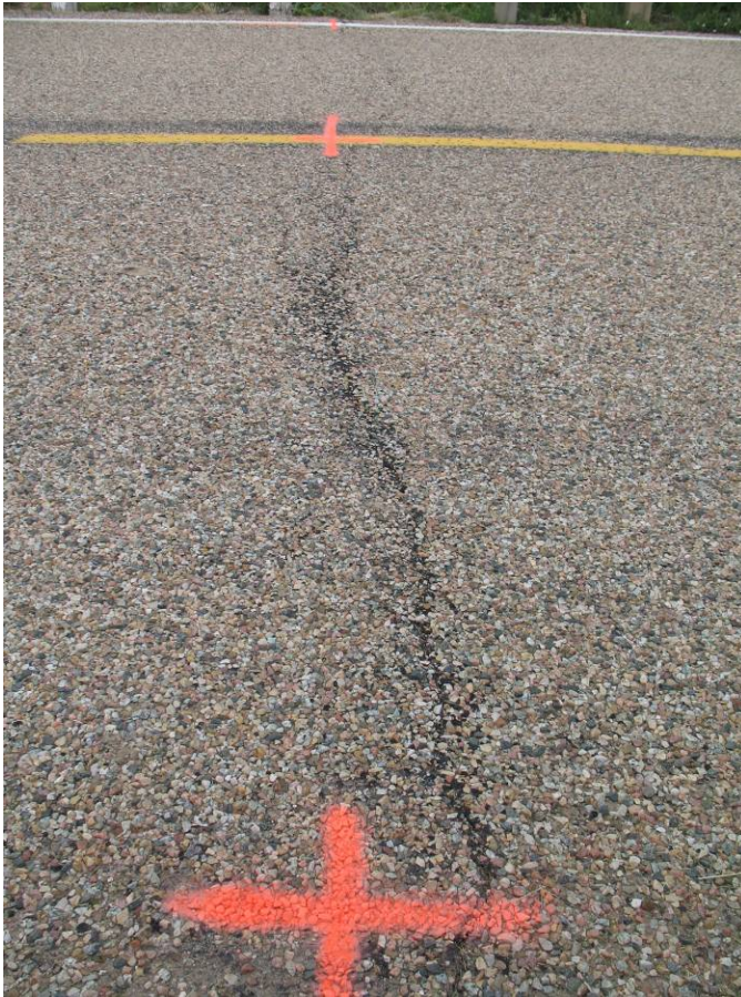
Figure 286. Transverse Wearing Surface Cracking
