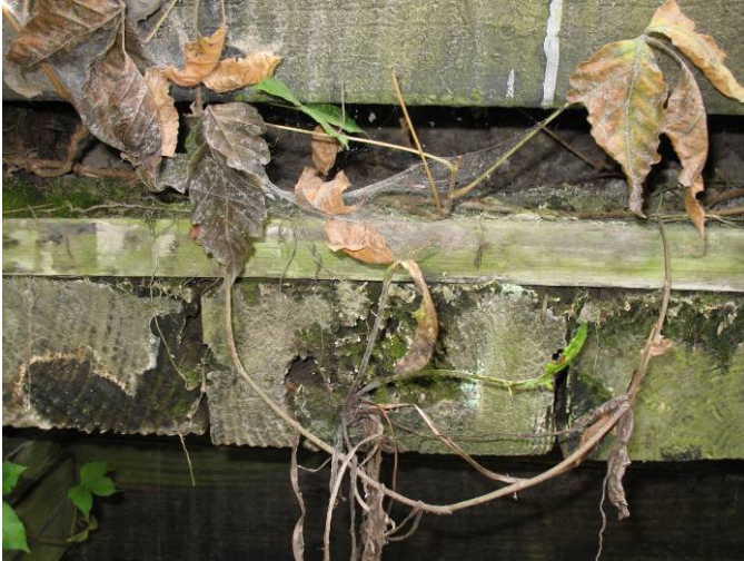
Figure 196. Decay in the Ends of the Deck Boards Superstructure
