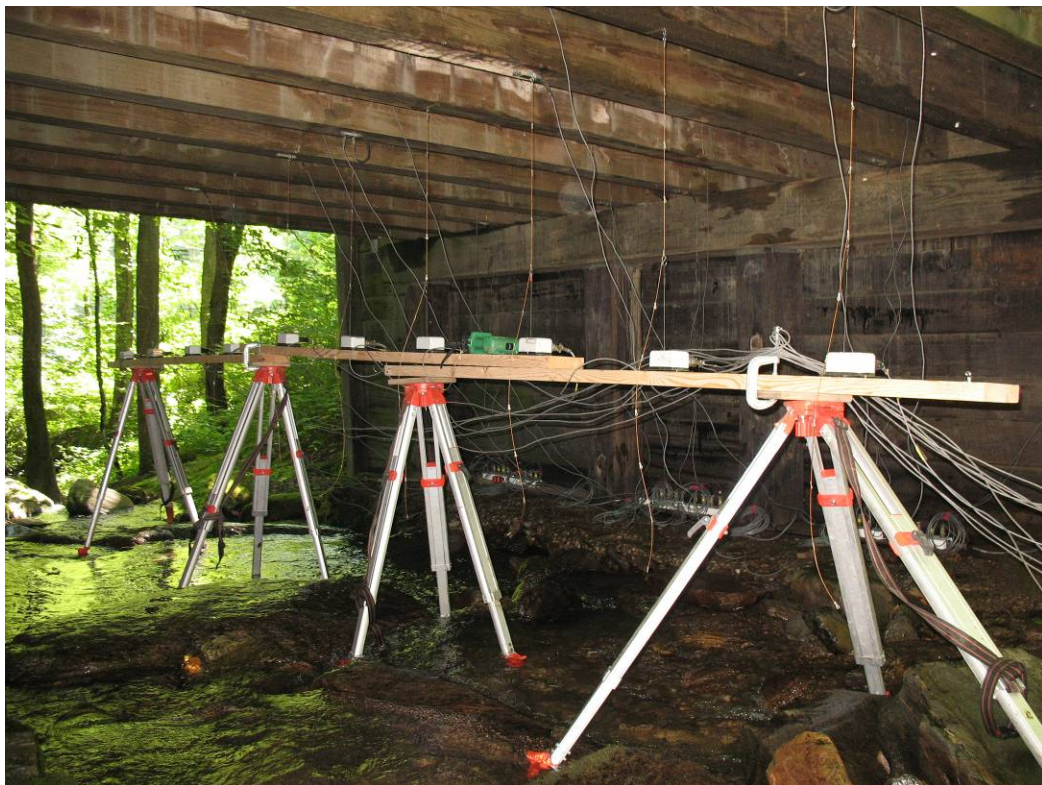
Figure 4. Typical Deflection Gage Instrumentation
