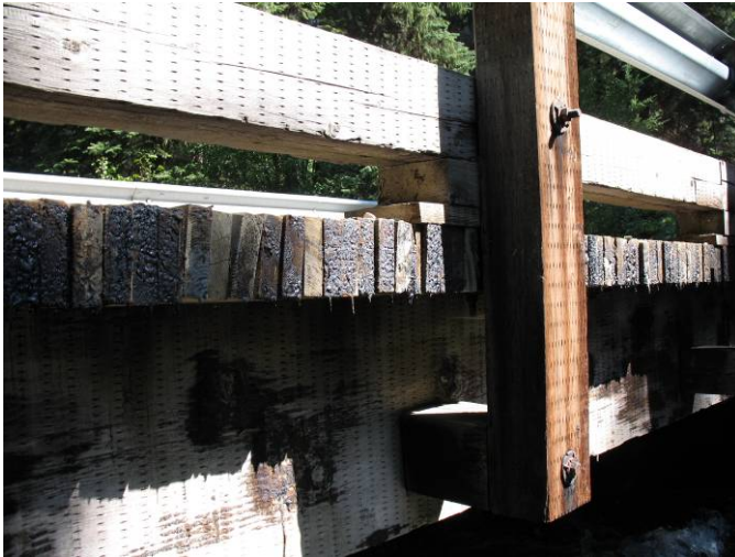
Figure 412. Twisting of Deck Boards
