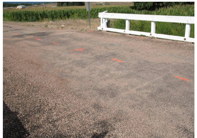
Figure 257. Transverse Wearing Surface Cracking
